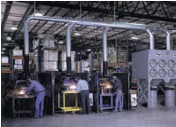
for welding smoke
